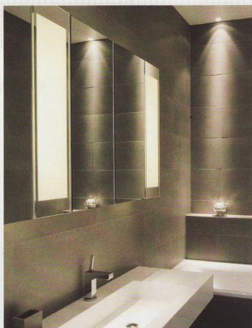
Sian Baxter Lighting Design set dimmable linear LEDs , £35-40 per m, behind frosted-glass doors.
